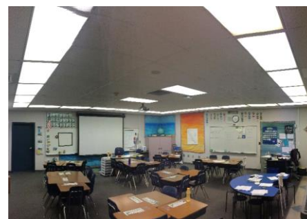
Figure 3: the original lighting system consisted of 26 fluorescent lights as shown above. Photo credit: PNNL
