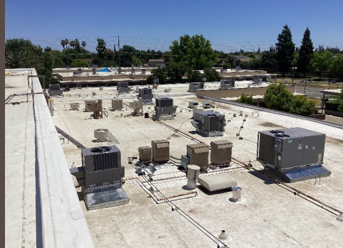
Capital Christian Center - HVAC
