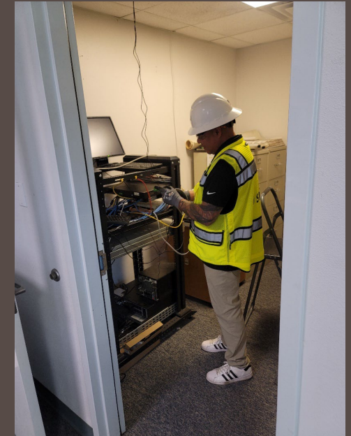
PowerDirect - Carmichael Water Treatment Plant
