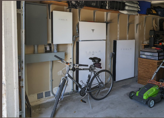
MEO Partner+ Tesla Battery installation
