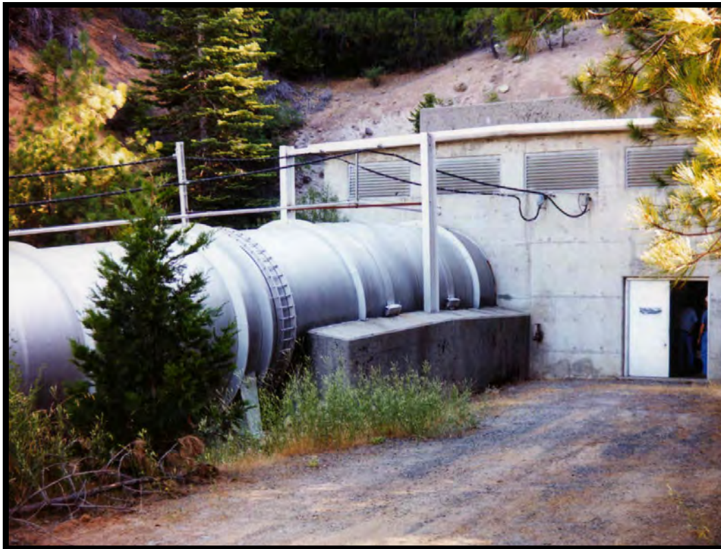
JB-5. Jaybird Valve House
