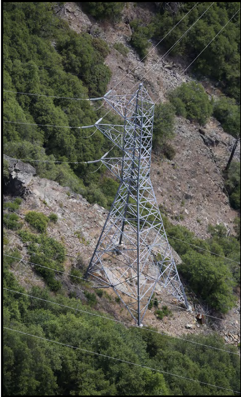
TL-6. Jaybird to White Rock Tower 230 kV
