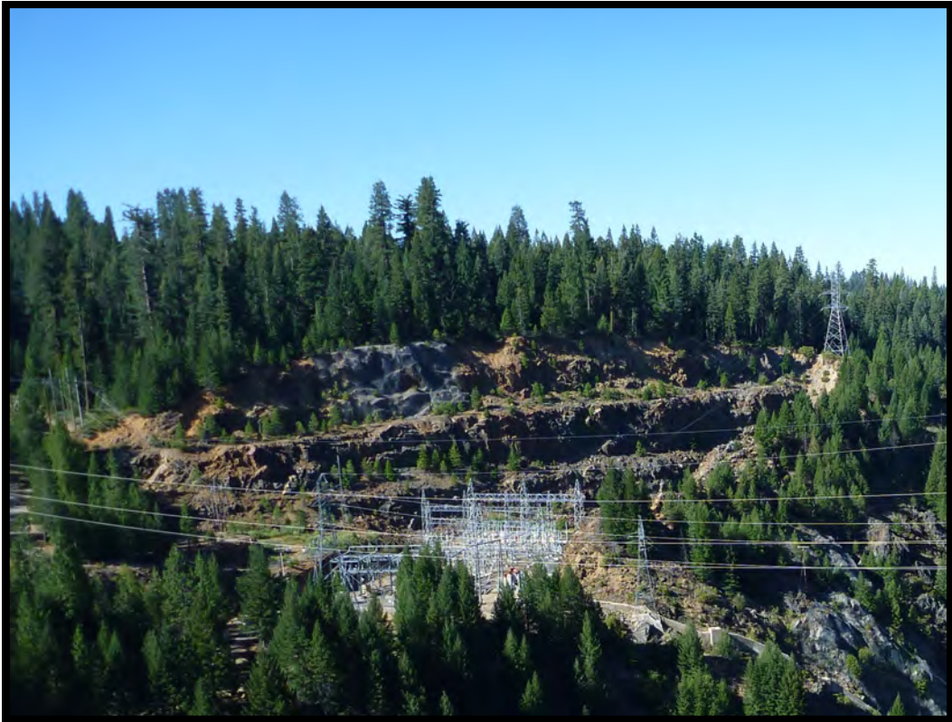
UV-4. Union Valley Switchyard
