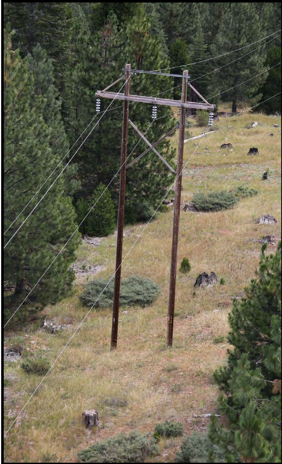
TL-4. Jones Fork to Union Valley 2-pole Tower 69 kV
