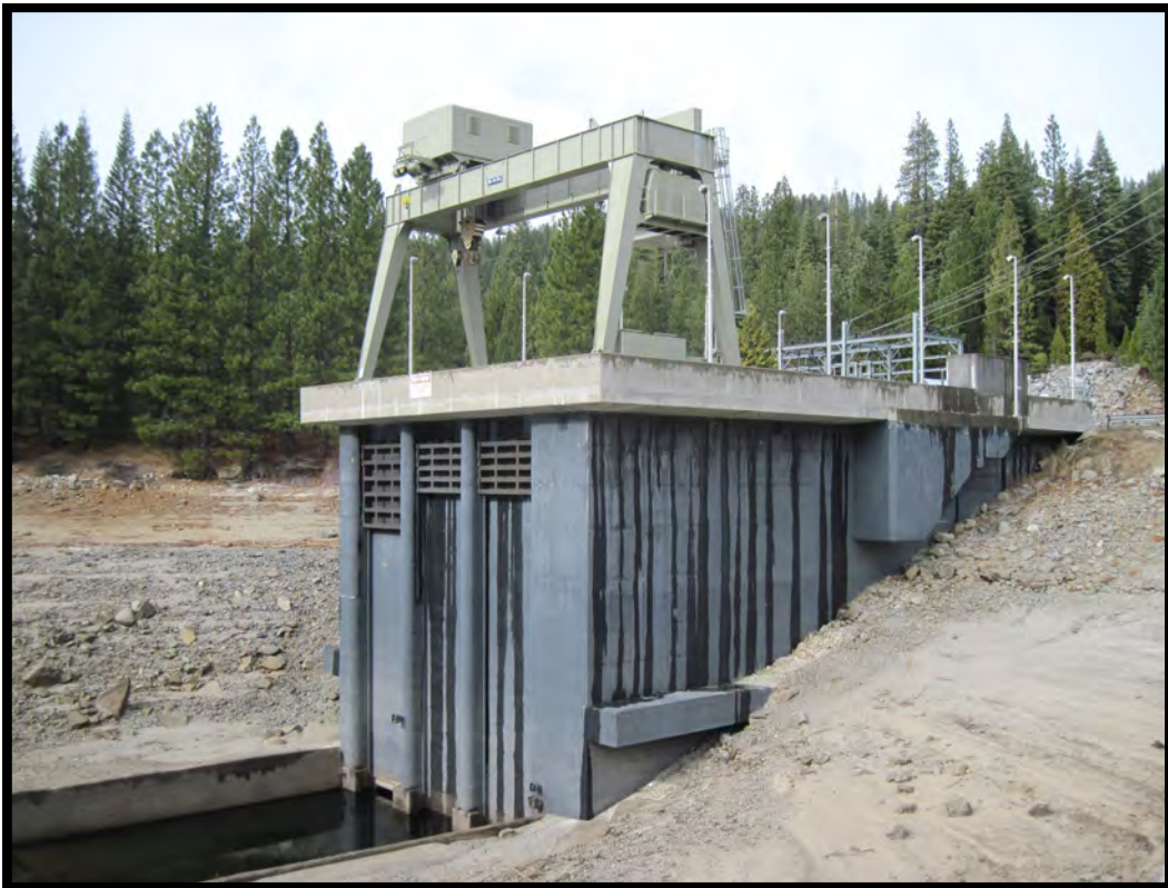
RP-6. Robbs Peak Powerhouse
