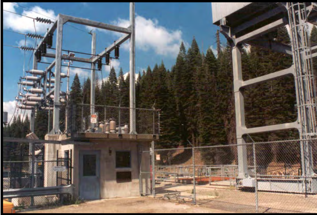
JF-3. Jones Fork Powerhouse and Switchyard
