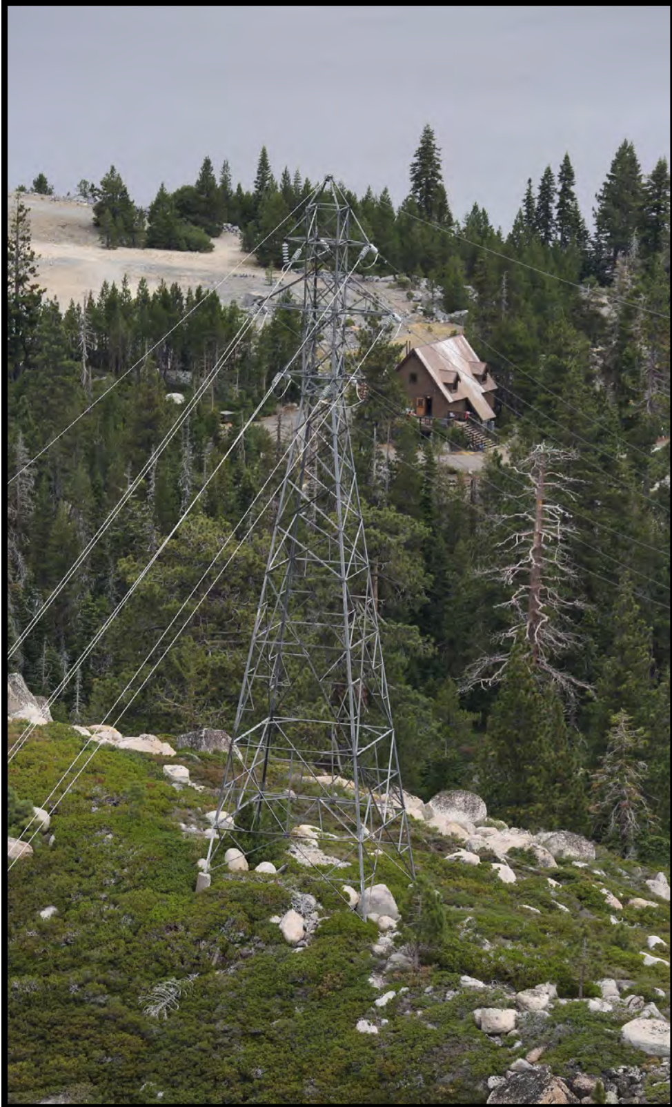
TL-1. Loon Lake to Union Valley 69 kV
