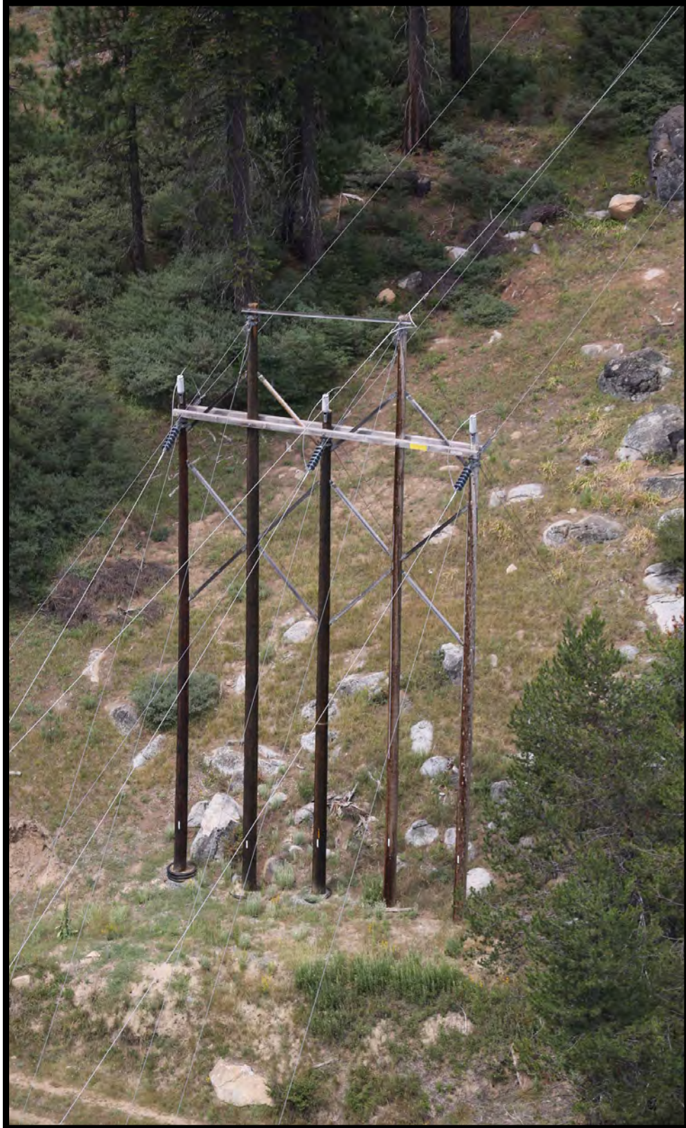
TL-3. Jones Fork to Union Valley 5-pole Tower 69 kV
