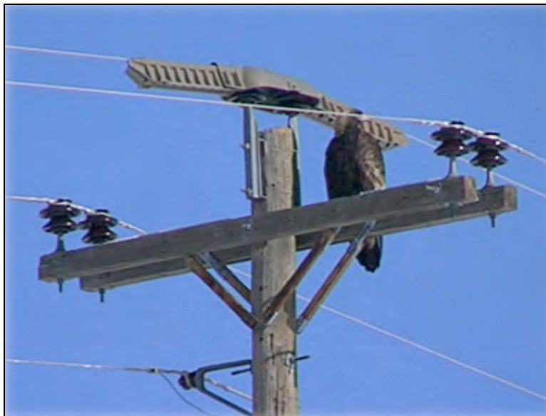
Exhibit 5-8. Example of conductor insulator on center conductor. No other modifications are required to make this pole configuration raptor safe. (Photo courtesy of Rick Harness and EDM International, Inc.)
