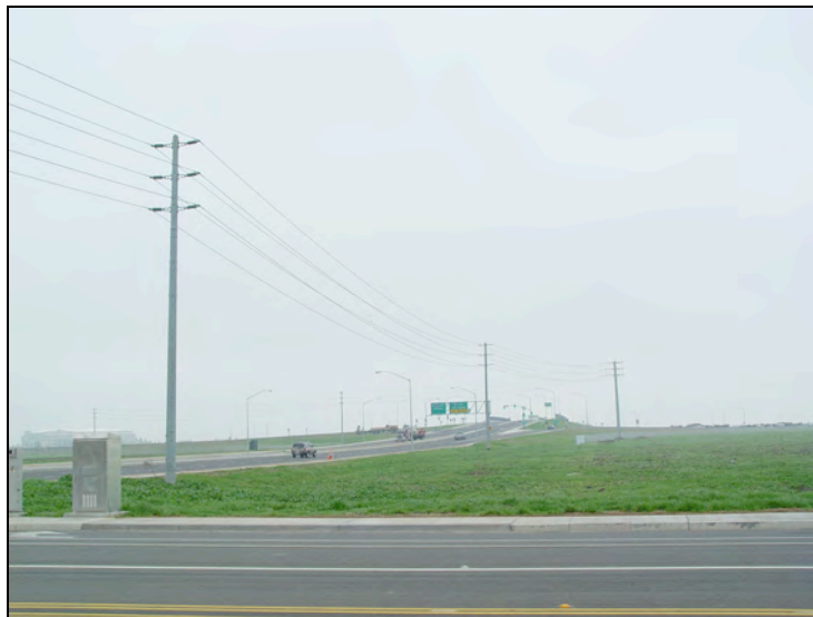
Exhibit 4-13. 69 kV (double circuit) power line.
