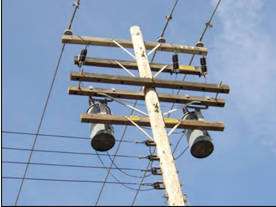
Exhibit 4-20. Double transformer bank.
