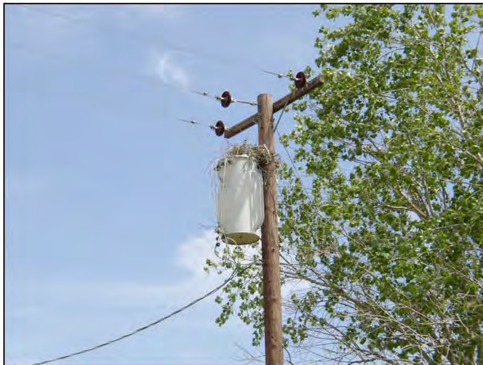
Exhibit 2-7. Red-tailed hawk nest on transformer.
