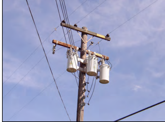
Exhibit 4-21. Triple transformer bank.
