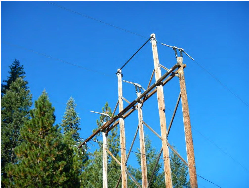
Photo 2. Type H 5-pole structure on the 69 kV Jones Fork line retrofitted with insulators.
