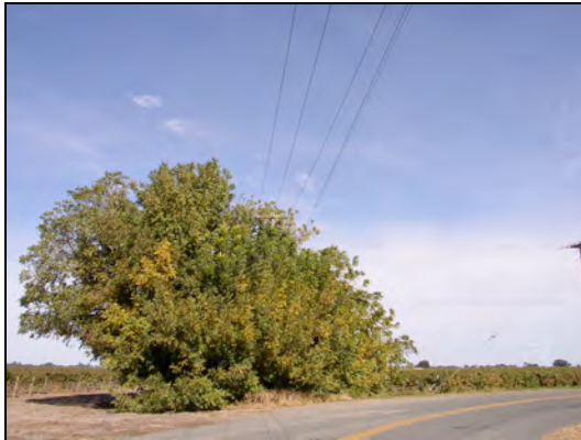
Exhibit 2-4. Conductors in vegetation reduce visibility.
