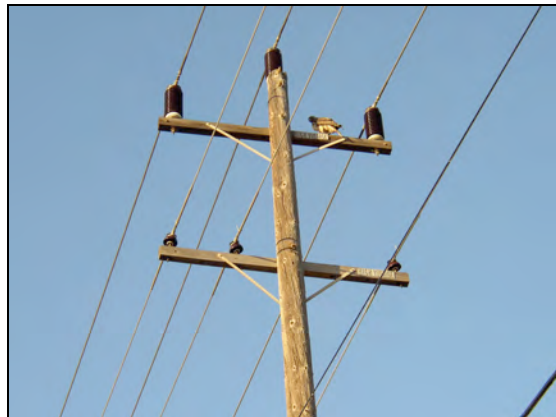
Exhibit 4-17. Double crossarm, three phase each; upper with center, lower with two on one.
