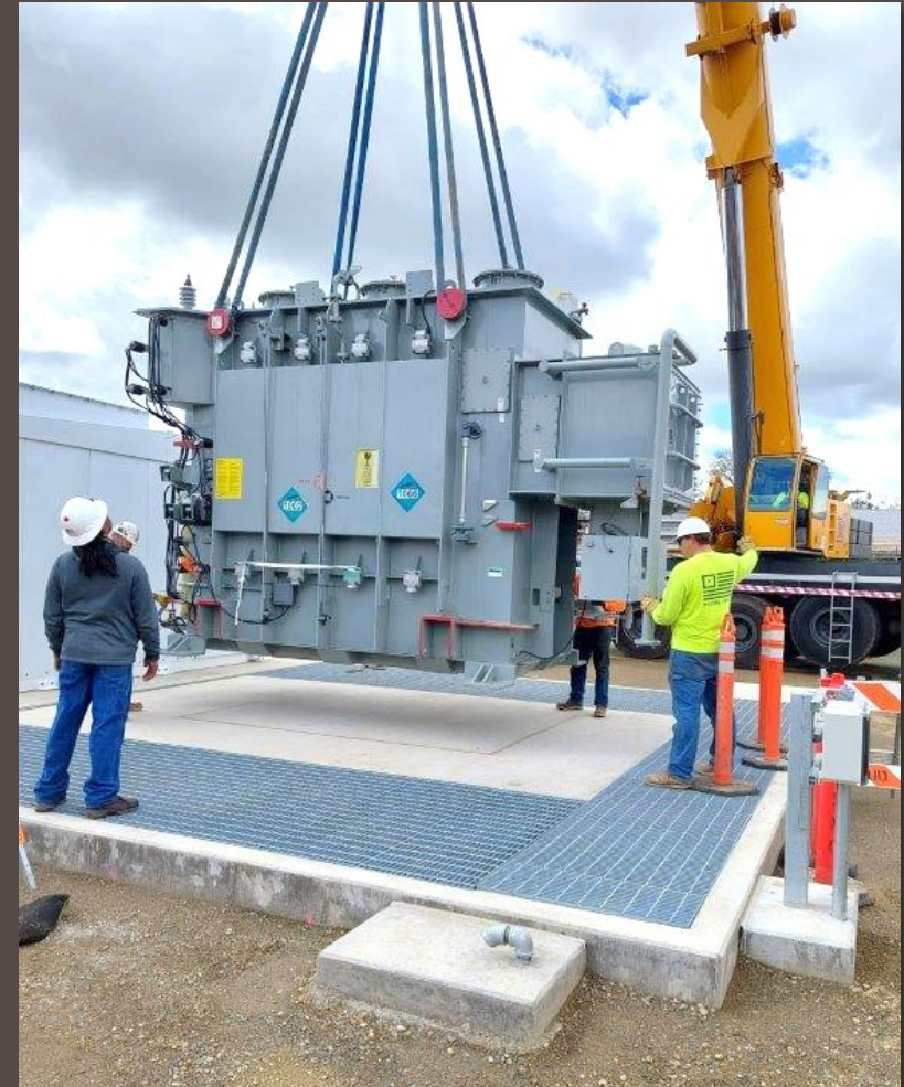
Requa Fawn Substation Transformer
