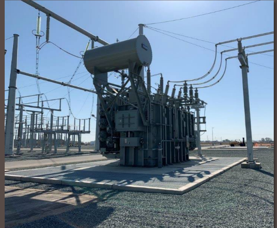
Franklin Bulk Substation Transformer
