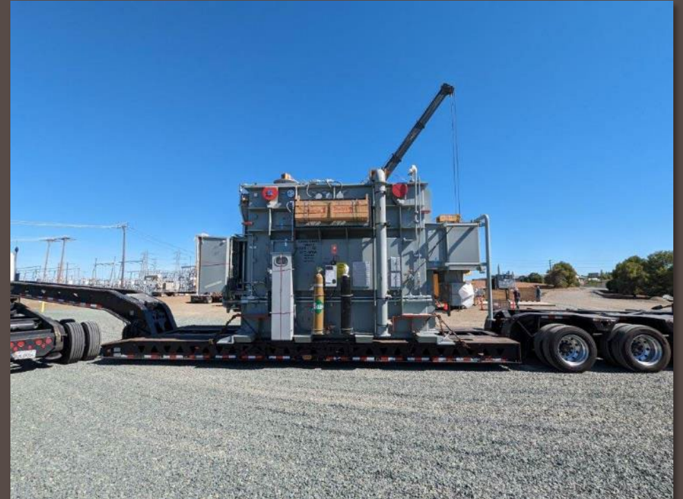
Station B Spare Transformer Delivery
