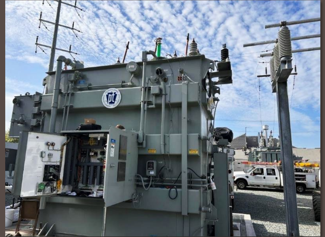
Sunrise Antelope Distribution Transformer
