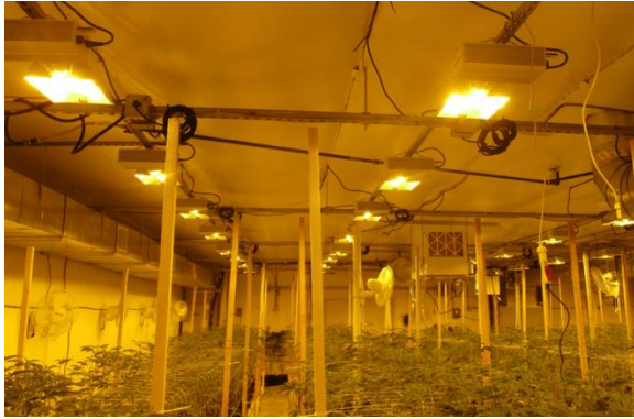
Figure 3: Nanolux HPS fixtures installed in Room 2.
