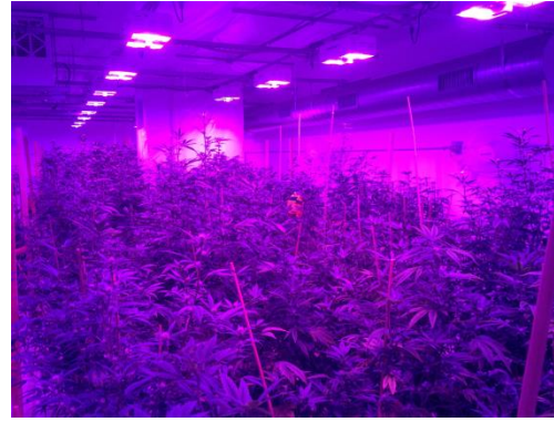
Figure 4: LumiGrow LED fixtures installed in Room 3.
