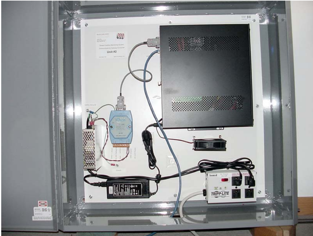
Figure 5-2 Data Acquisition and Communications Gateway Box
