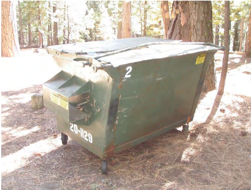
Photo 7. Bear-proof trash receptacle with missing clip and cable, bent bar and no pad.
