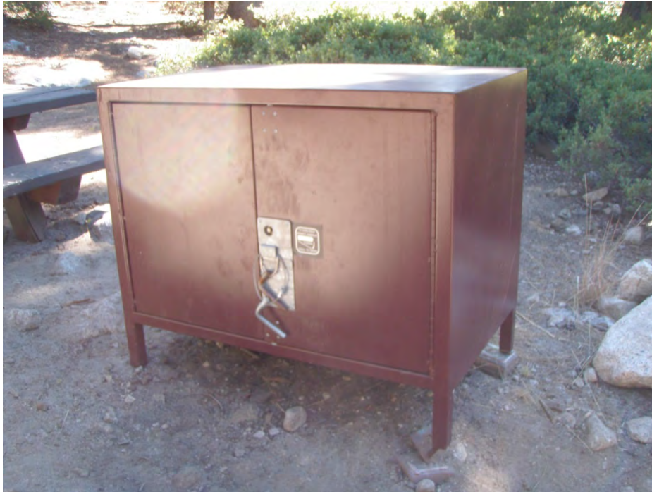
Photo 10. Bear-proof locker in good cosmetic condition with original latch broken and unstable footings.
