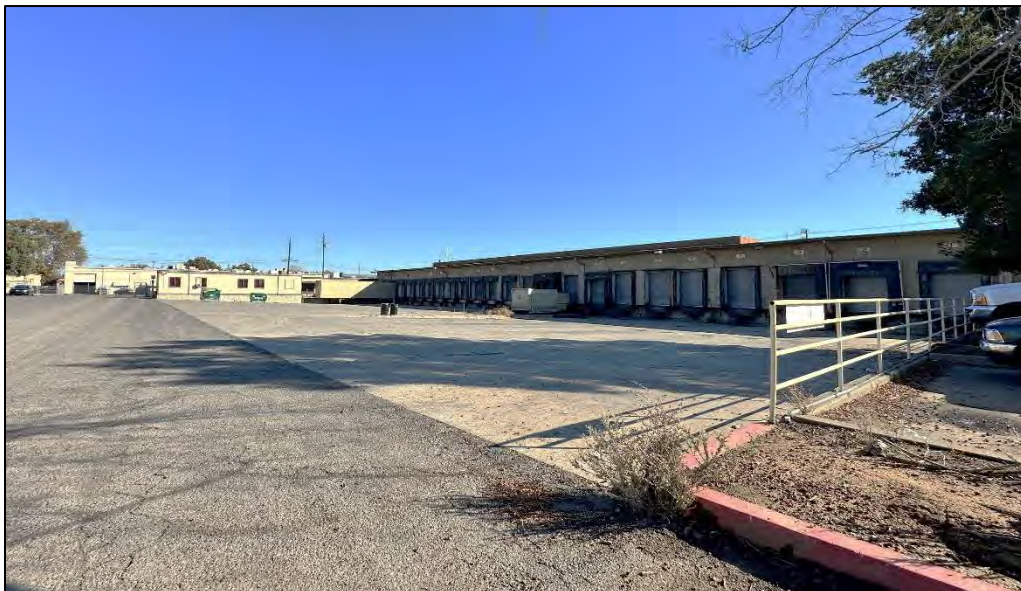
Photograph 5: West elevation of warehouse with 22 bays along the loading dock with slanted pavement, camera facing northeast, November 10, 2022.
