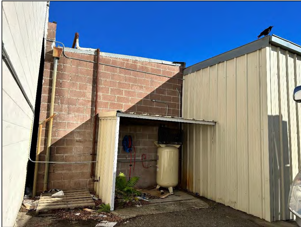
Photograph 4: Air compressor concrete block enclosure at south end of building and other additions, camera facing northeast, November 11, 2022.
