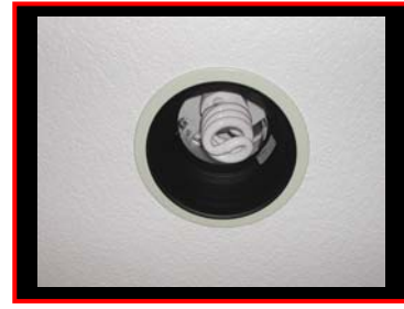
Screw-in compact fluorescent installed in a conventional recessed downlight
