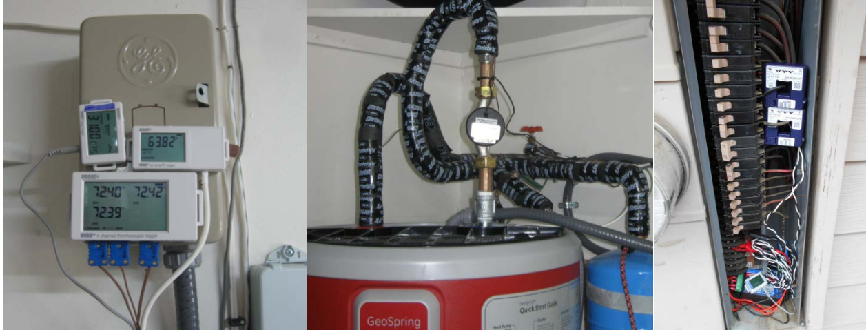
Figure 5: Pictures of Metering Equipment in Place: Loggers (Left), Water Flow Meter (Middle), Power Meter (Right)
