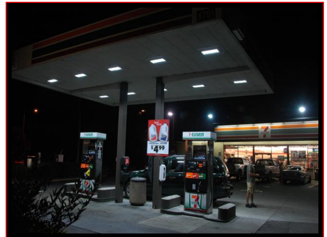
Figure 2: The new LED lighting system for the fueling canopy area included ten recessed, 115-Watt LSI Crossover fixtures. Photo: Stephen Anselmino
