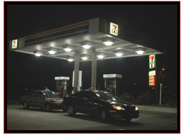
Figure 1: The original exterior lighting system for the fueling canopy area included ten surface-mounted, 250-Watt metal halide fixtures. Photo: Stephen Anselmino
