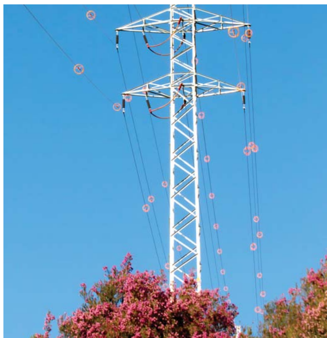
Flight diverters on powerlines
