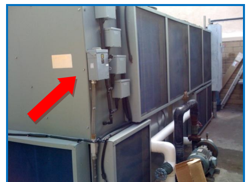
Figure 2: water control valve boxes.
