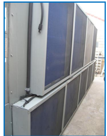
Figure 1: evaporative cooling pads.
