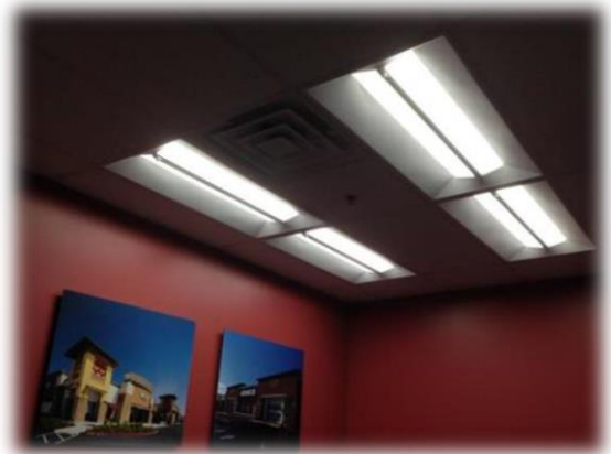
Figure 4: New LED Lighting Fixtures
