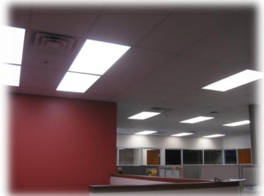
Figure 2: Original Fluorescent Lighting Fixtures
