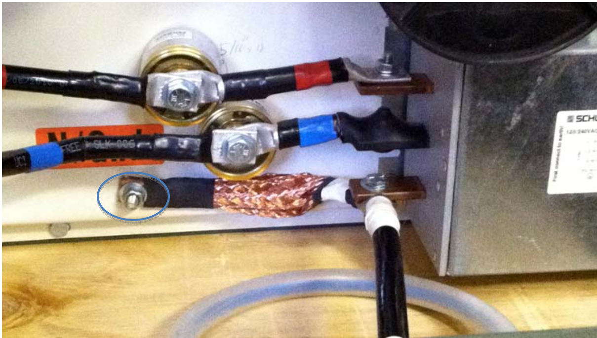
Figure 5. Detail of neutral wire connection. The bolt indicated by the circle is the location for connecting the wire to the driven ground in the pad of the unit.
