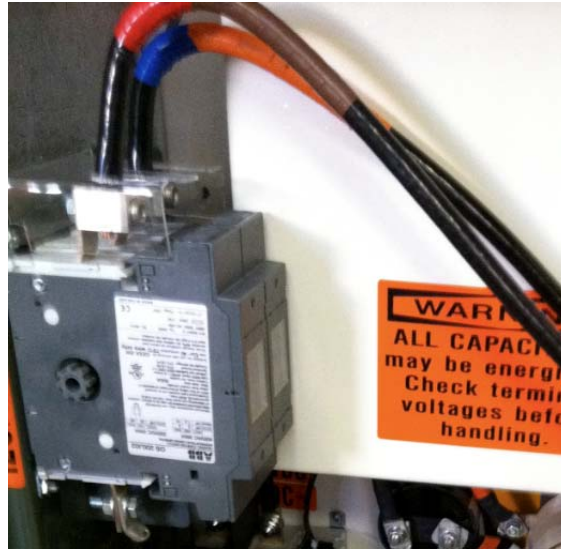
Figure 4. Detail of L1 and L2 connection to fused switch disconnect. This disconnect is the ON/OFF control for the CES and the only operable external control for the unit.
