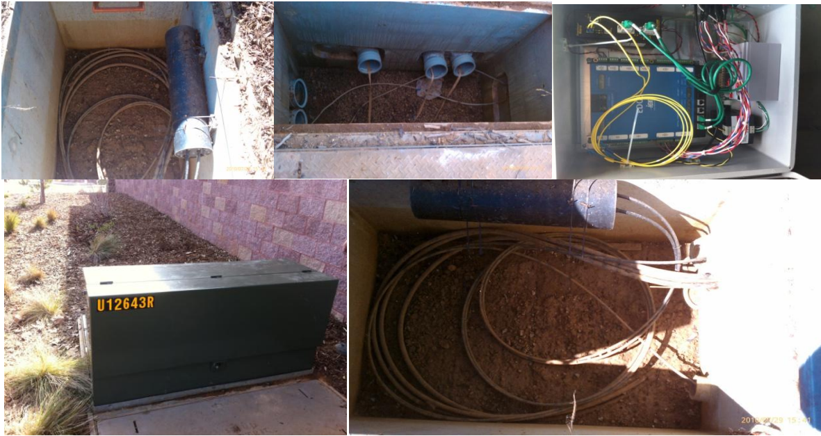
Figure 8. Pictures from Feeder Monitoring Installation
