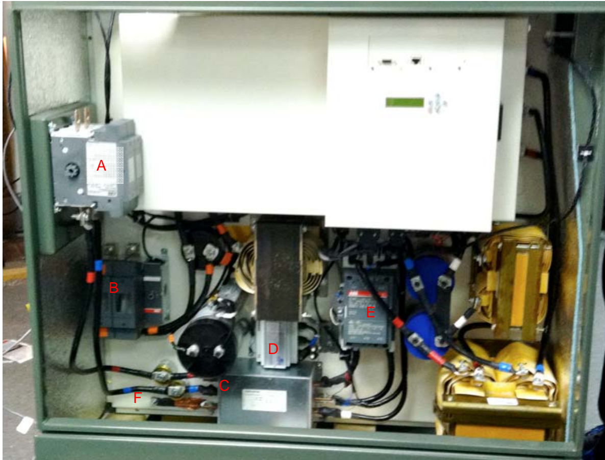
Figure 2. Photograph of internal construction of the PCS portion of the CES unit. (A) AC-side fused switch disconnect (ON/OFF control), (B) DC-side fused switch disconnect, (C) EMI filter, (D) Current probe amplifier, (E) AC contactor, (F) single grounding point connection.
