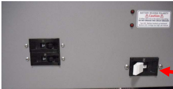
Circuit Breaker Panel
