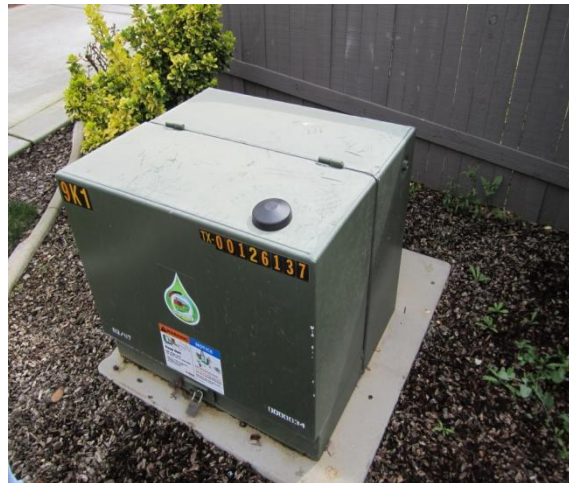
Figure 10: DMU Installed on 9K1
