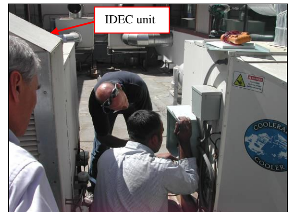
Figure 7: Crew installing the controls for the new unit. Note the IDEC immediately next to the Coolerado.
