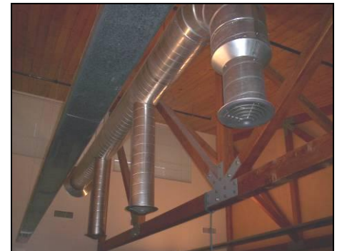
Figure 10: The project team decided to install new ductwork for the Coolerado. Photo credit: ADM Associates Inc.
