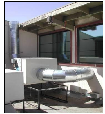
Figure 6: The first Coolerado was installed at ABC School in 2004.
