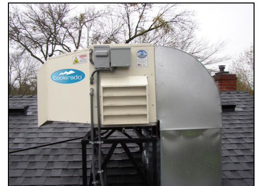
Figure 20: Coolerado R400 at Site 2.
