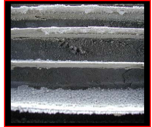
Scale formations in a cooling tower. Photo provided courtesy of BWI Solutions Inc.
