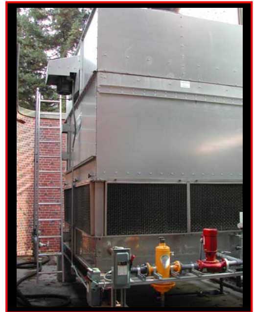
Cooling Tower for Rodda Hall North
