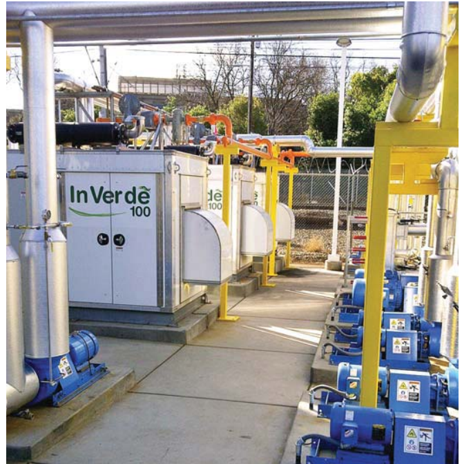
Installed Tecogen Inverde 100 natural gas engines and related equipment
