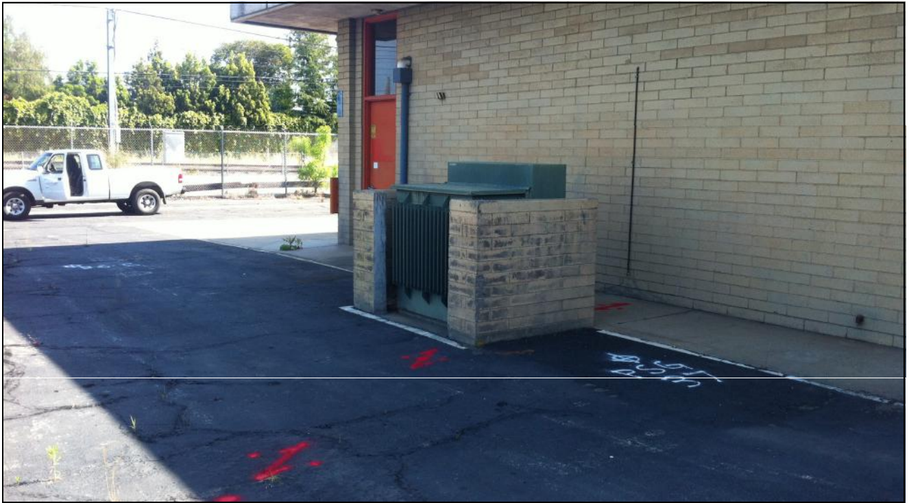
Image 47: PSG-37 is located west of the Pre Fab Building at the South Corporation Yard
