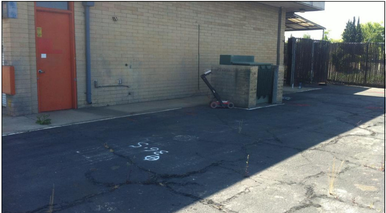
Image 46: KA-36-S is located west of the Pre Fab Building at the South Corporation Yard
