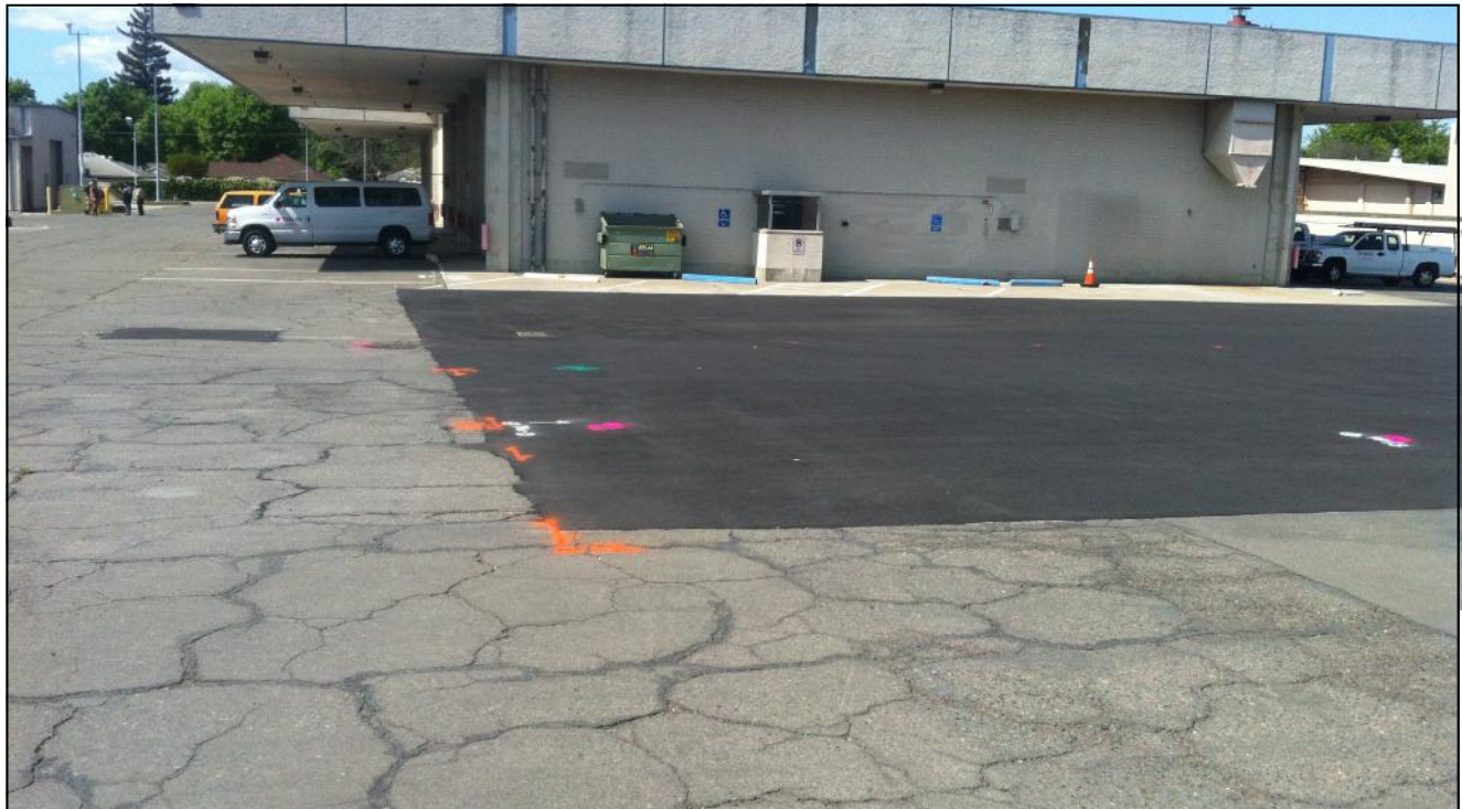
Image 12: PSG-8 and KA-1-S are located in former UST area west of the Garage Building
