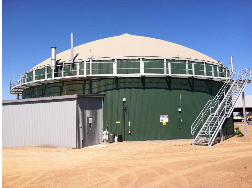
Figure 4-1: New Hope Tank Digester
