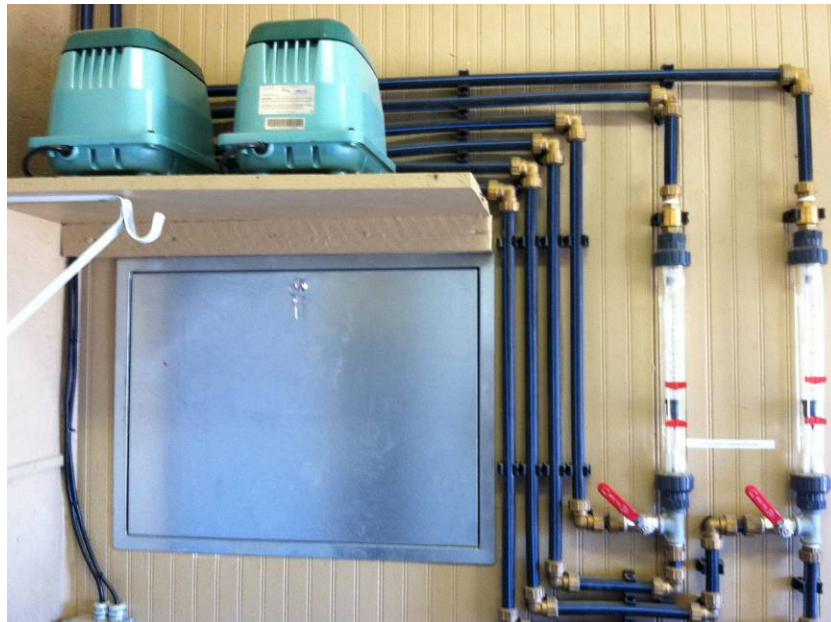
Figure 6. Air Injection System for H 2 S Reduction in Control Room
