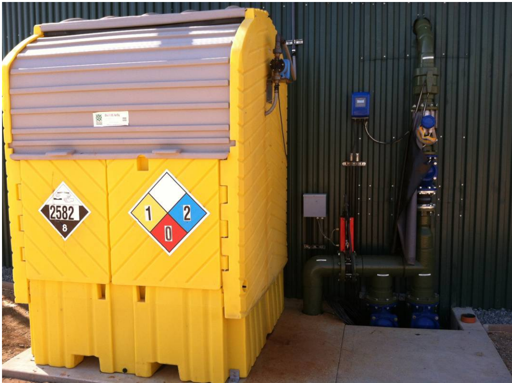
Figure 3 Ferric Chloride dosing system and Influent pipes entering digester.
