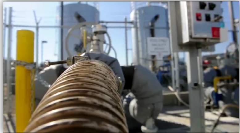
Figure 5 – Unloading Station and BEP Tanks
