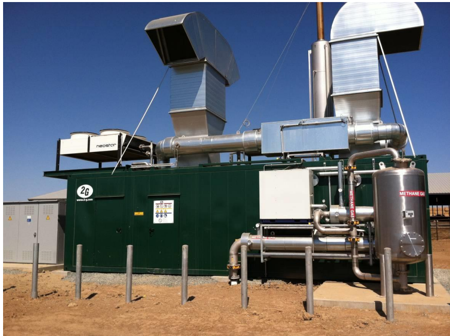
Figure 4-2: New Hope 450 kW Engine-Generator
