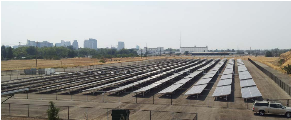
Figure 6. Photograph of the ground-mounted system
