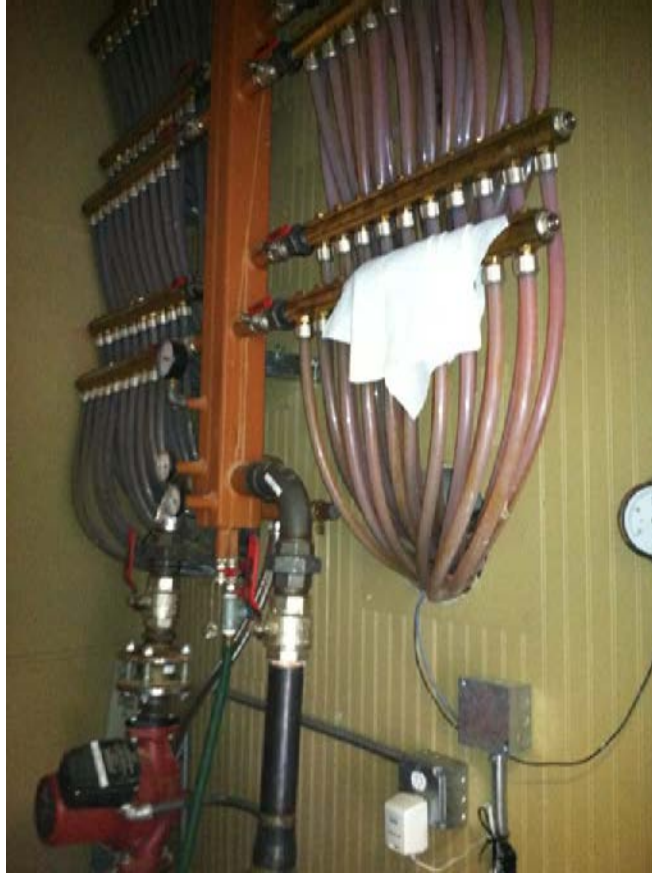
Figure 5. Hot water pipes for digester heating in control room
