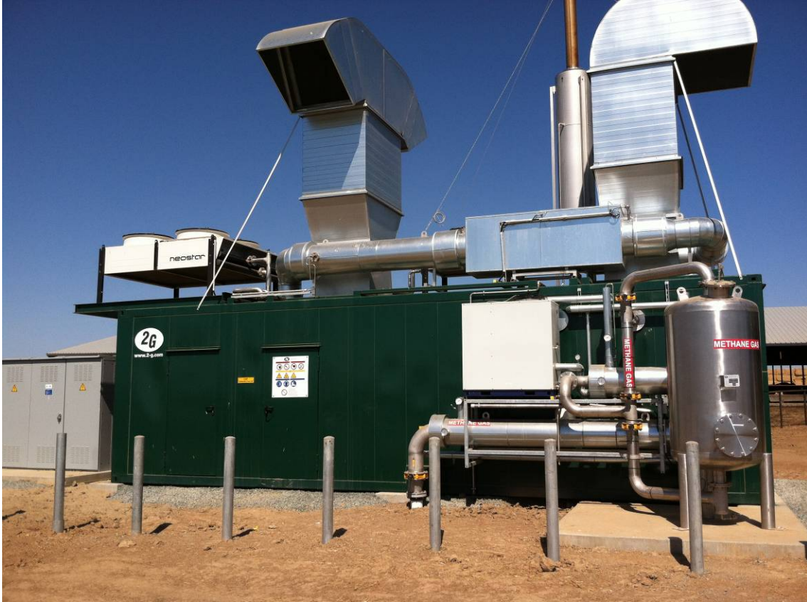
Figure 7. New Hope Dairy 450 kW engine-generator
