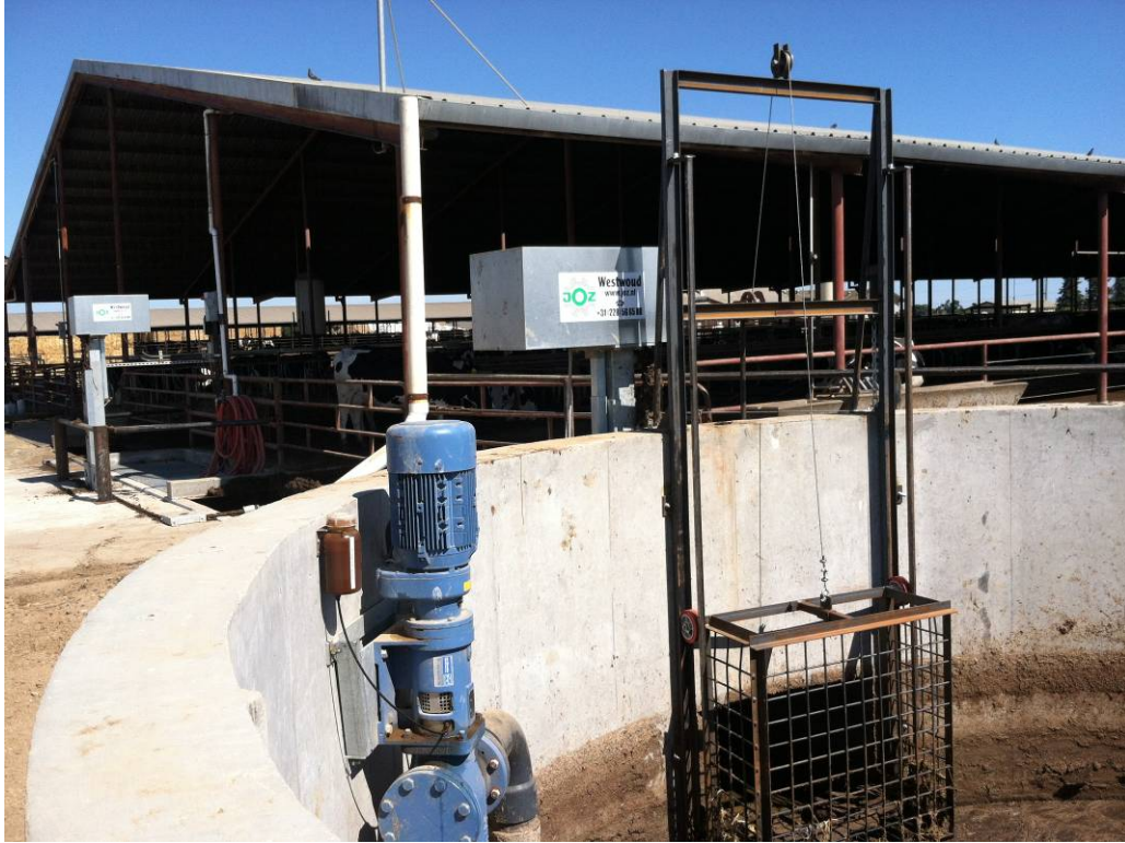
Figure 2. Manure slurry collection tank.
