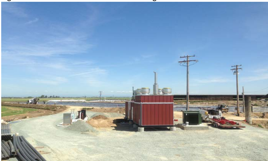
Figure 1: Genset Container and Covered Lagoon
