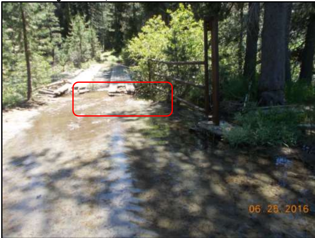
Figure 11. Erosion of bridge approach on Parcel H, at about 375 cfs
