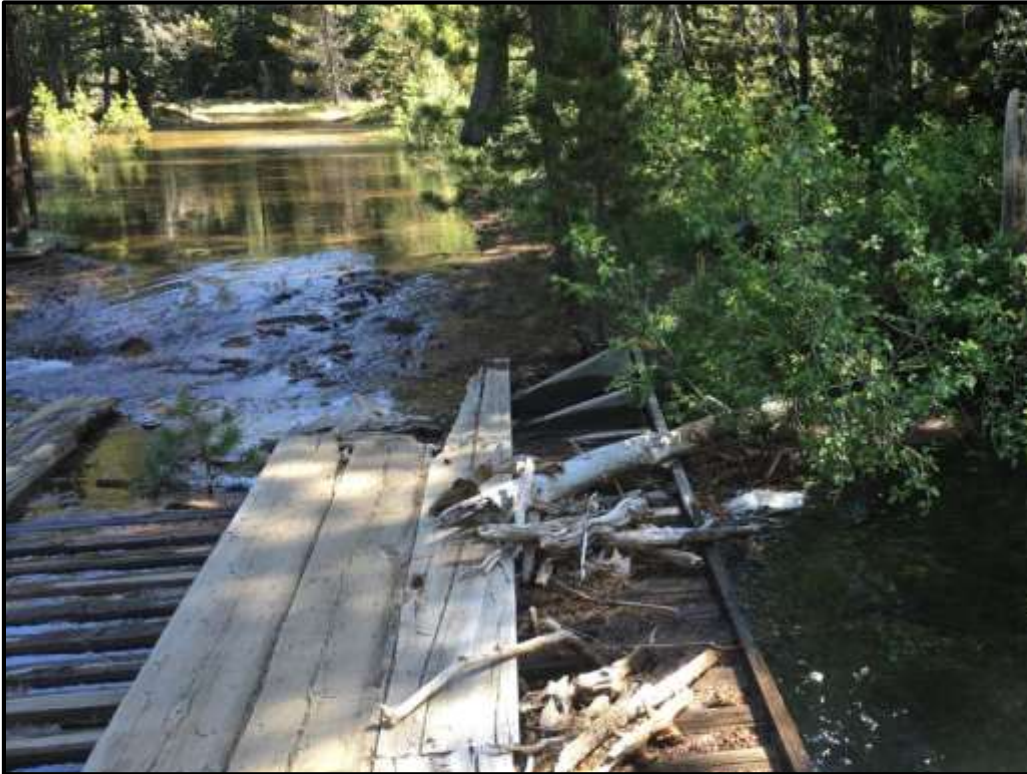
Figure 4. Erosion of bridge approach on Parcel H, 6/3/16, at about 500 cfs
