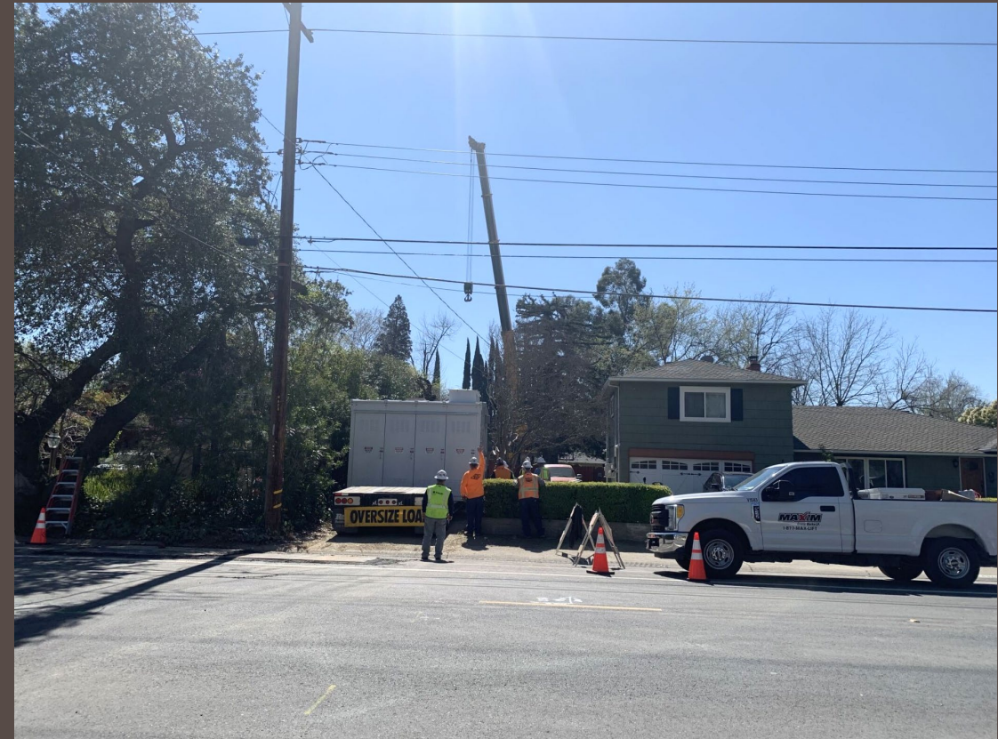
Engle Eastern Substation Switchgear
