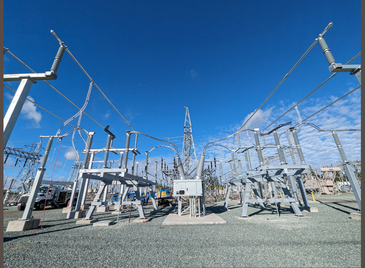
Hurley Substation Bus Tie
