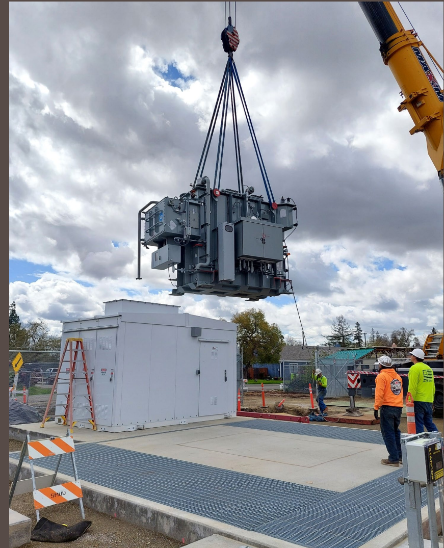
Transformer at Requa Fawn Distribution Substation
