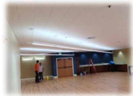
Figure 6: Philips BoldPlay indirect/direct LED fixtures (suspended)
