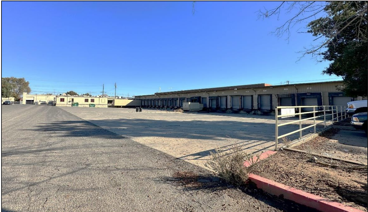
Photograph 3: West elevation of warehouse with 22 bays along the loading dock with slanted pavement, camera facing northeast, November 10, 2022.
