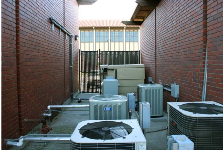
Figure 4. Ice Bear ® System installation at Sacramento City College
