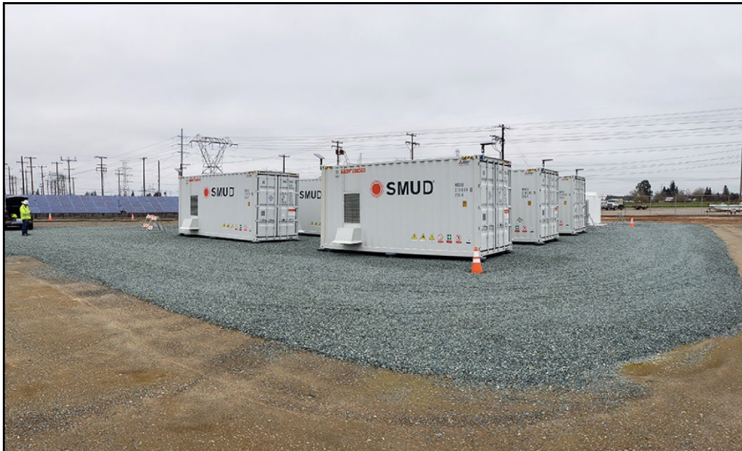
Figure 7. Battery Energy Storage System
