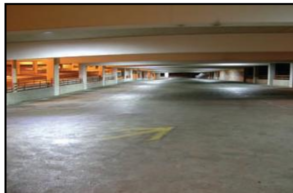
Figure 1: photos of the CSUS parking garage before and after the LED retrofit.
