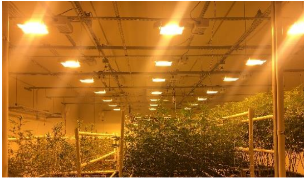
Figure 3: Nanolux HPS fixtures installed in Room 1.
