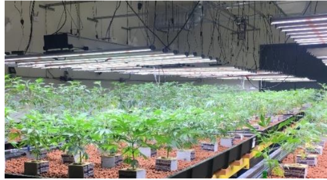
Figure 4: Fluence LED fixtures installed in Room 2.
